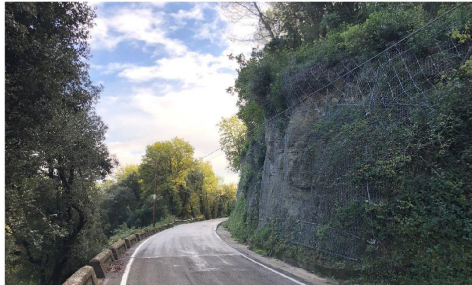
Talussos de roca alts i verticals
